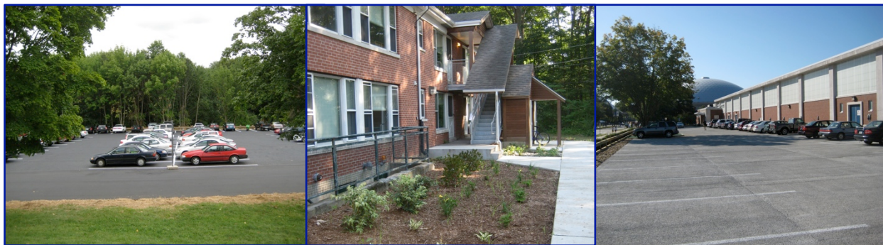
LID projects on campus. Left: Towers parking lot repaved with porous asphalt. Center: all buildings in the Northwoods Apartment complex have rain gardens to accept roof runoff. Right: porous concrete parking lot at the UConn Field House.
